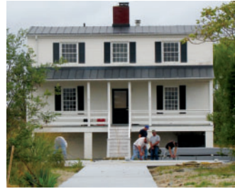
1) The former museum in the south campus area, damaged by Hurricane Isabel in 2003, is demolished. 2) Crews install curbing for the new museum entrance. 3) Workers install a new boardwalk made of recycled plastic in the south campus. (Photos by April Havens)
